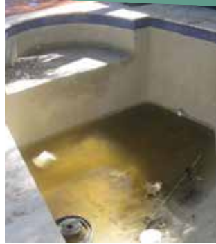
Stagnant pooling water
